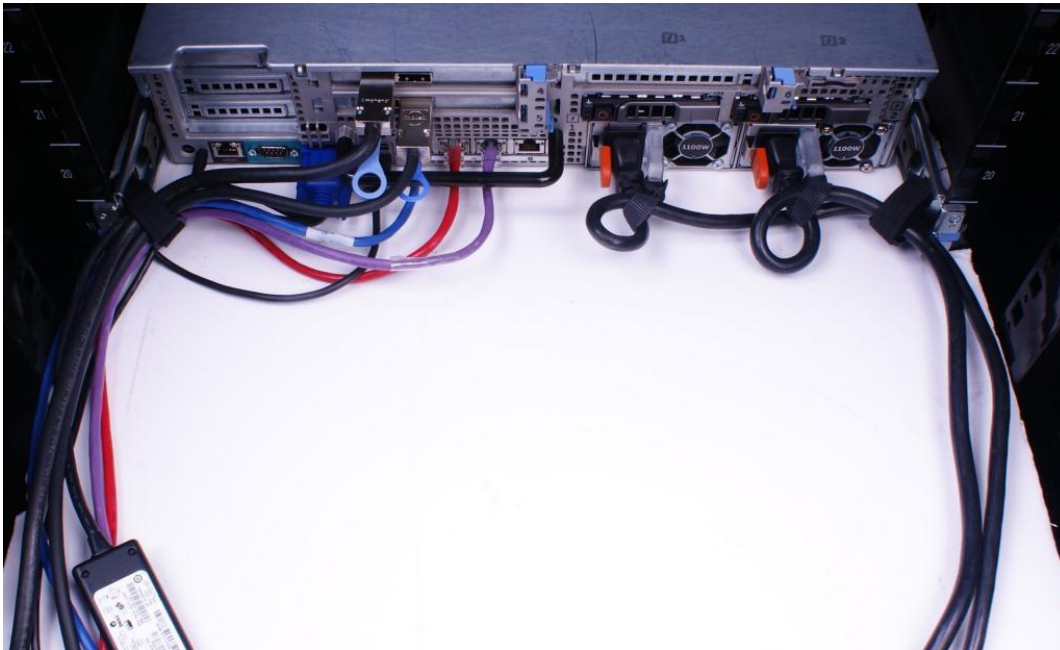
Figure 11. Cabling a system installed in static rails
